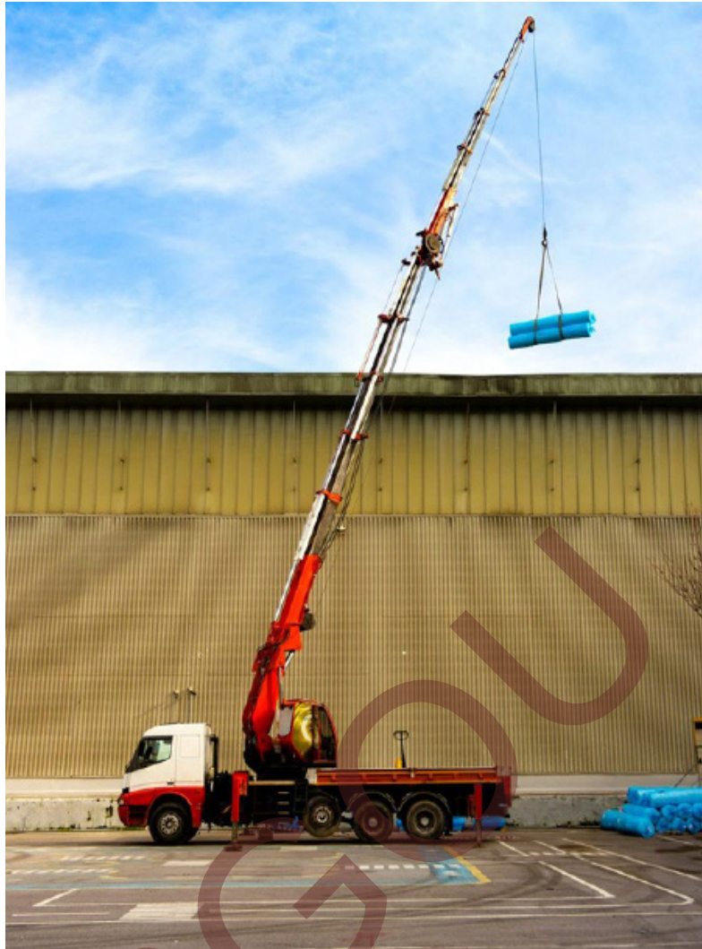
Fig. 5.2.8 Mechanical handling equipment
