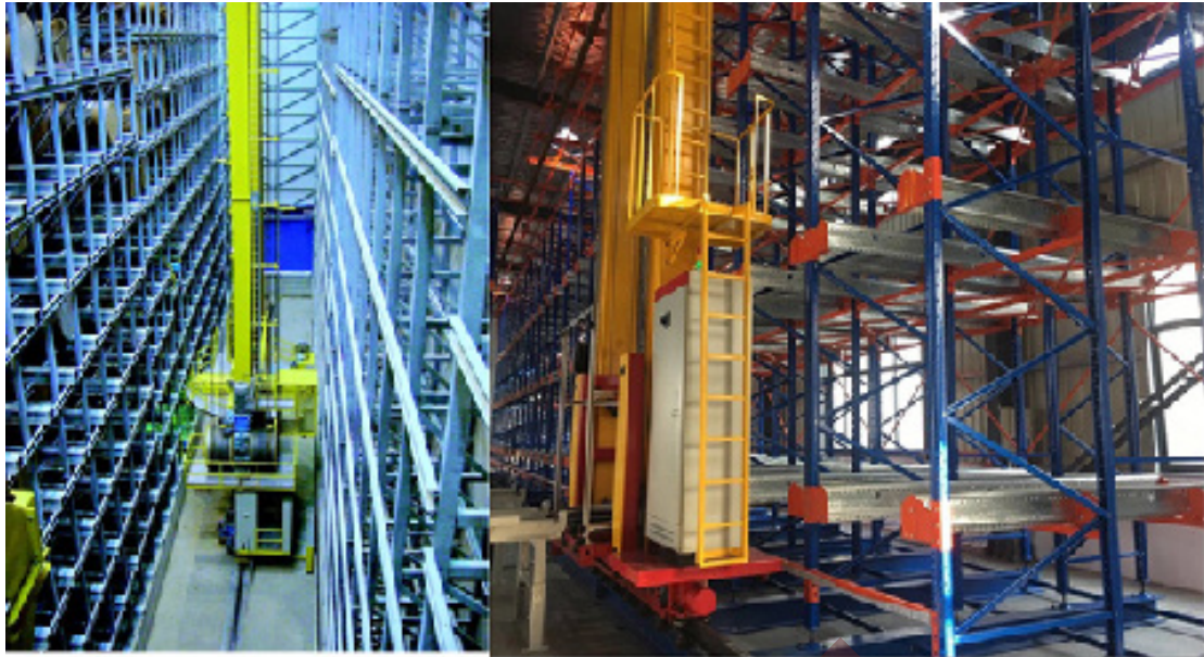
Fig. 5.2.5 Automated Storage and Retrieval Systems (AS/RS)
